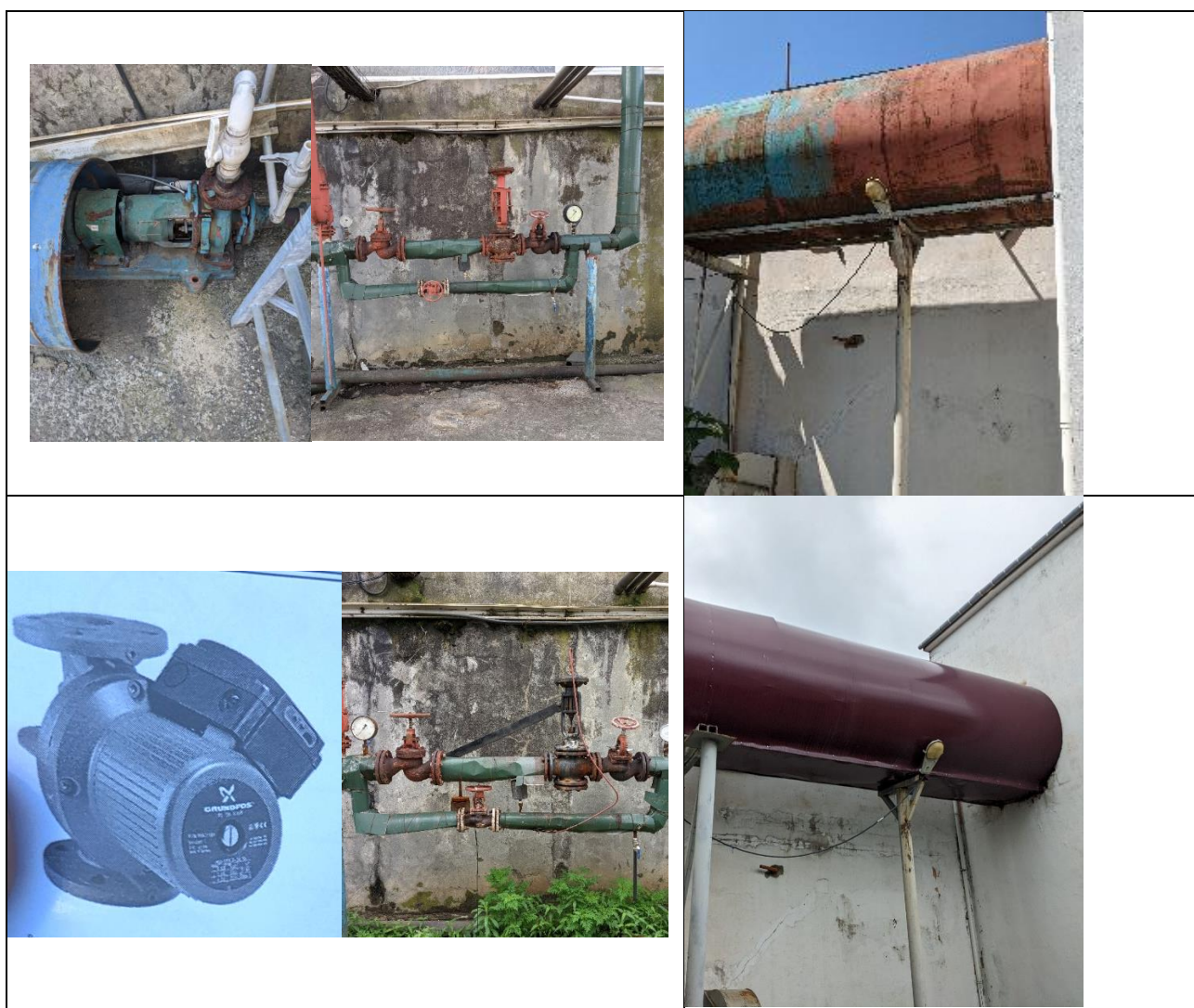
Figure 2. Condensate circulator pump, pressure regulator valve and condensate tank before and after the implementation of RECP measures
